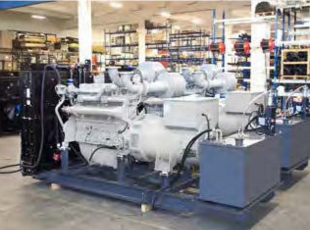
800 KVA WITH DOUBLE WALL TANKS 1000 LTS
