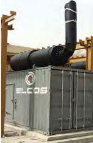
FAR EAST POWER PLANT 3 X GENSETS IN CONTAINER 2
