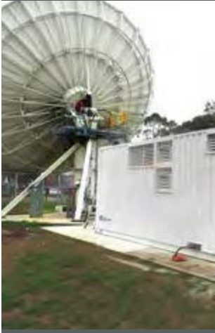
AUSTRALIA SATELLITE PLANT 2 X GENSETS IN CONTAINER 2
