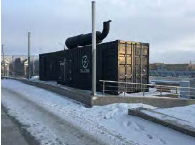
KAZAKHSTAN GENSET IN CONTAINER 40'1880/1700 kVA
