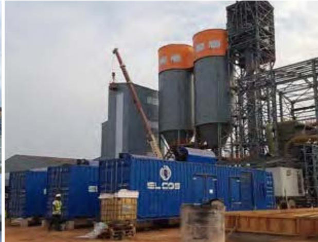
SOUTH AFRICA POWER PLANT 3 X GENSETS IN CONTAINER
